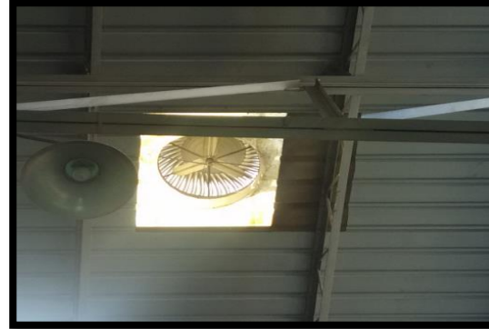
2. NATURAL AIR: USE OF TURBO VENTILATORS AND TRANSPARENT SHEETS THROUGHOUT FACTORY ROOF.
