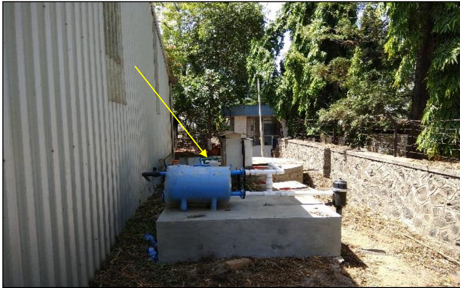
Reuse of ETP processed water for gardening with the help of drip irrigation @ 5-6 KL per day
