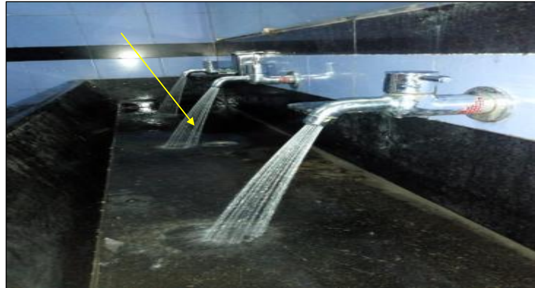
Installation of water saving sprinkler nozzle for water taps - Saving 300 ml water per use
