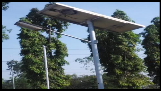
1. SOLAR LAMPS IN FACTORY PREMISES. TOTAL 9 NOS.
